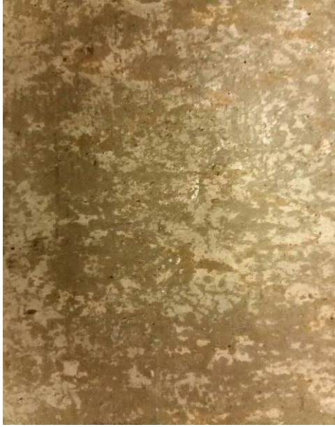
Figure 4.30a: Concrete column subject to 100% relative humidity
